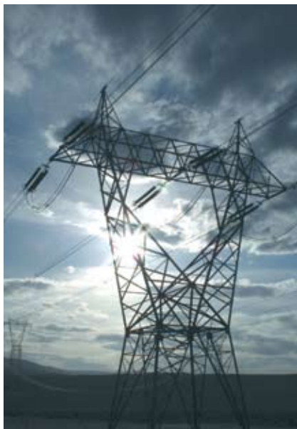
High-voltage transmission lines in Washington state. Higher voltage lines are more susceptible to geomagnetic storm damage.
