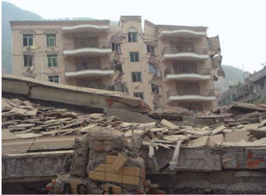
Damage to the Agriculture Development Bank of China branch in Bei Chuan after the devastating earthquake, May 12, 2008. The U.S. Geological Survey reported that there were “at least 69,195 people killed, 374,177 injured and 18,392 missing and presumed dead in the Chengdu-Lixian-Guangyuan area. More than 45.5 million people in 10 provinces and regions were affected. At least 15 million people were evacuated from their homes and more than 5 million were left homeless. An estimated 5.36 million buildings collapsed and more than 21 million buildings were damaged.... The total economic loss was estimated at $86 billion.”
